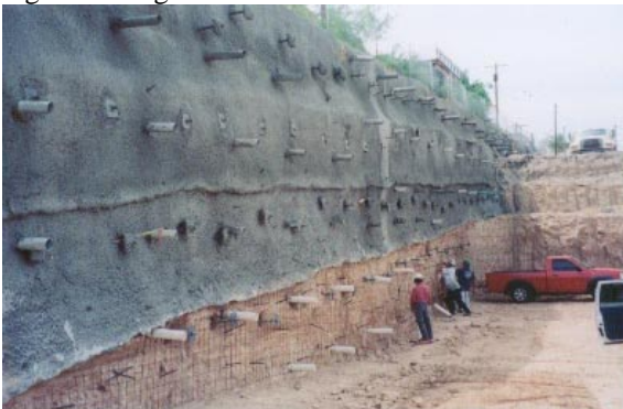
Photo 1-47 New retaining wall under construction using helical tension anchors as soil nails.
