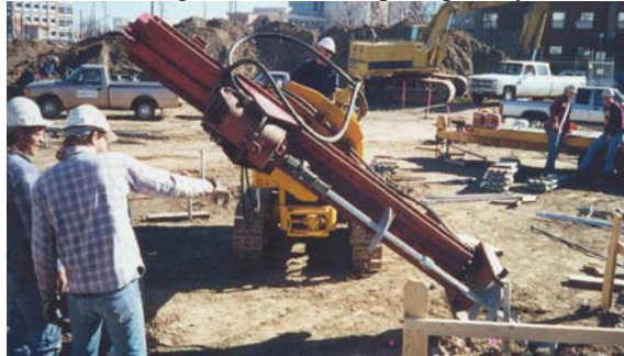
Photo 1-52 Tracked machine with adjustable frame installing battered helical piles for lateral loads.
