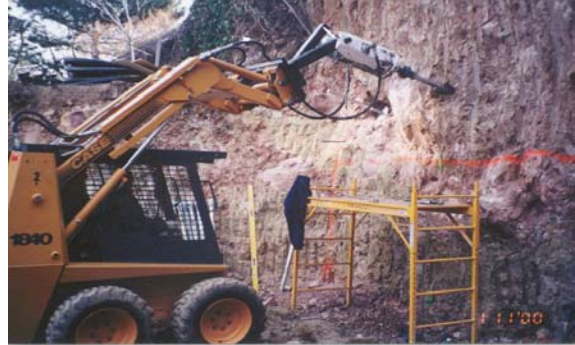
Photo 1-74 Skid-steer machine installing helical tension anchors as tiebacks for new retaining wall.
