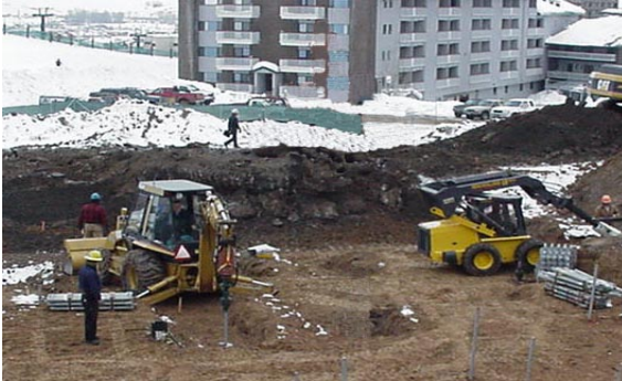
Photo 1-73 Skid-steer machine (on right) installing helical tension anchors as tiebacks for structure.
