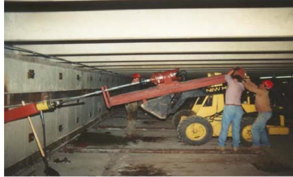
Photo 1-76 Skid-steer mounted drive head installing helical tension anchors as tiebacks in low overhead.
