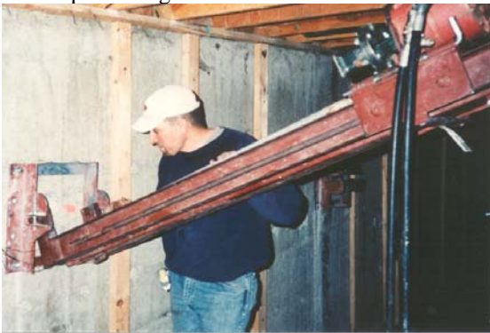
Photo 1-69 Hand-carried mast in near horizontal position to install helical tiebacks in low overhead.
