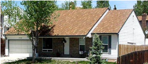
Photo 1-27 Existing residence with 18 inches differential heave in expansive soil underpinned and stabilized with helical piles.
