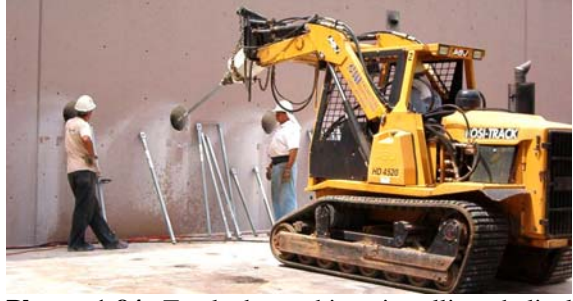
Photo 1-84 Tracked machine installing helical tension anchors as tiebacks for retaining wall repair.
