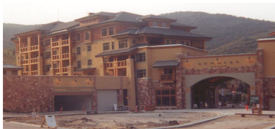
Photo 1-32 Existing building still under construction settled. Foundation underpinned and stabilized with helical piles.
