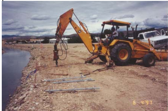
Photo 1-82 Backhoe mounted torque motor installing helical screw piles at a slight batter for a sound wall.
