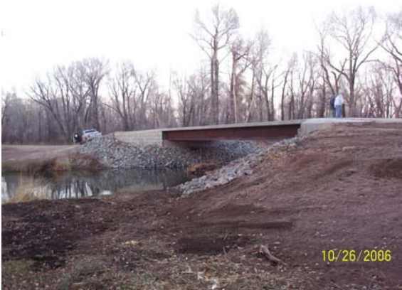
Photo1-35 New steel bridge with abutments supported on helical piles and helical tiebacks.
