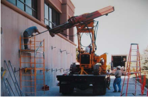
Photo 1-71 Tracked machine to install helical tension anchors as tiebacks for retaining wall repair.
