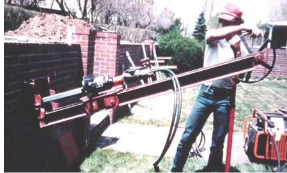
Photo 1-78 Hand-carried mast in near horizontal position installing helical tension anchors as tiebacks.
