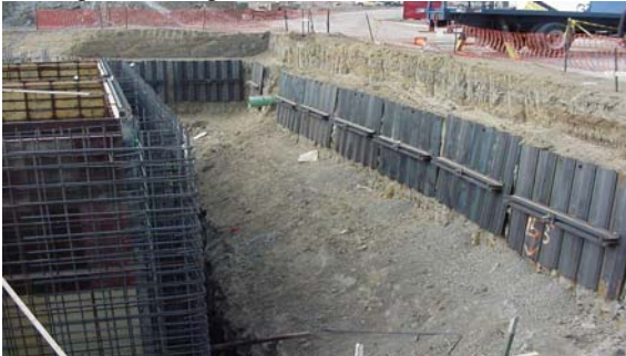
Photo 1-45 New pre-engineered shoring panel shoring wall using helical tension anchors as tiebacks.
