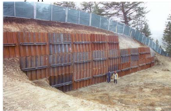
Photo 1-48 New pre-engineered shoring panel shoring wall using helical tension anchors as tiebacks.
