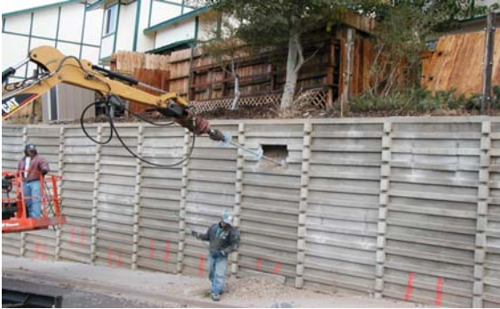
Photo 1-75 Backhoe mounted torque motor installing helical tension anchors as tiebacks for repair.
