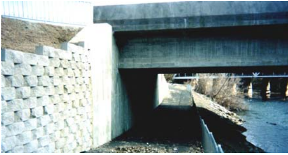
Photo 1-33 New reinforced concrete multi-lane bridge with abutments supported on helical piles and helical tiebacks.
