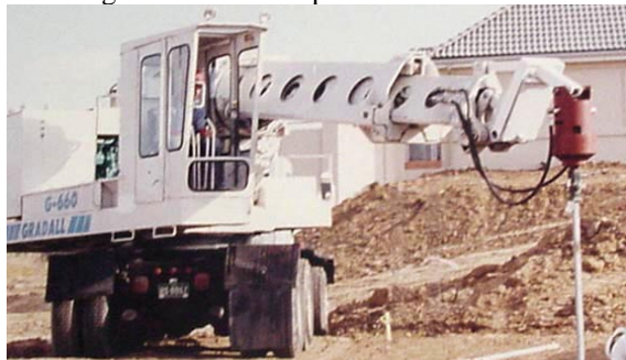
Photo 1-54 Rubber-tired hydraulic excavator is capable of installing over 60 helical piles per day.
