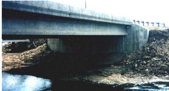
Photo 1-34 New reinforced concrete multi-lane bridge with abutments supported on helical piles and helical tiebacks.
