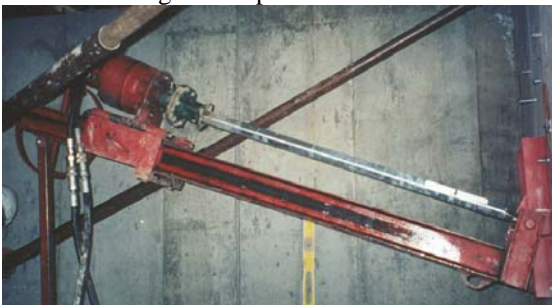
Photo 1-93 Hand-carried mast mounted on wall in near horizontal position to install helical tiebacks.
