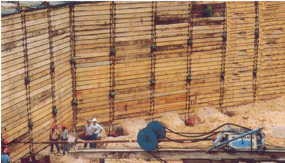
Photo 1-43 New soldier beam and wood lagging shoring wall using helical anchors as tiebacks.
