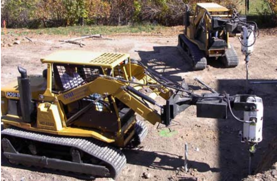
Photo 1-51 Two tracked machines each capable of installing over 60 helical piles per day.
