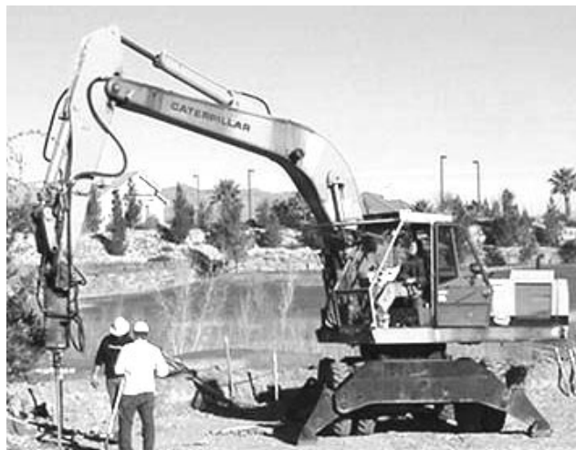
[Paper No. 2] Figure 5. Square Shaft Helical Pier Installation in Expansive Soils. 40,000 lb (178 kN) Machine
